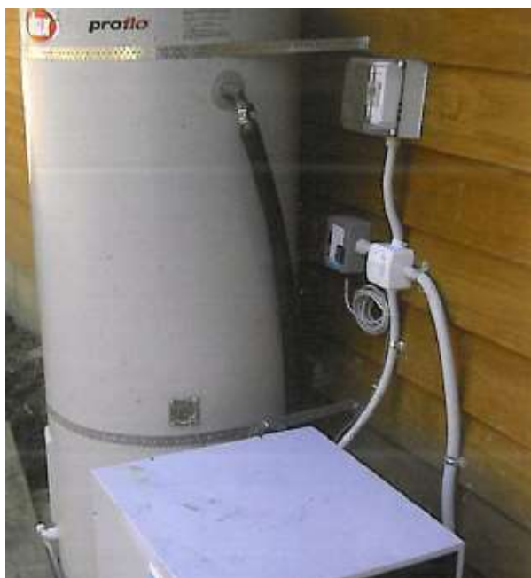
A split heat pump hot water system – the cylinder can be inside the house.
